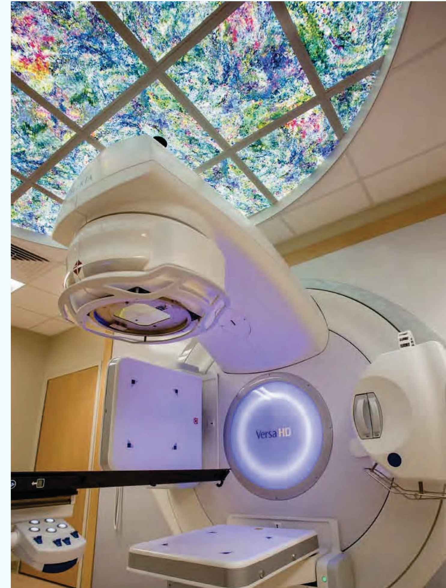
William E. Kahlert Regional Cancer Center Linear Accelerator Suite Westminster, MD “Infinite Moments”
